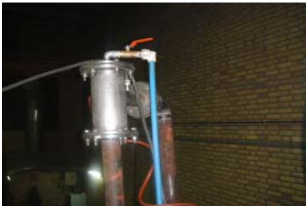
Figure 10. Hydro cyclone installed on pilot system
