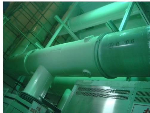
Figure 1. The bus ducts of IPB Pars Generator
