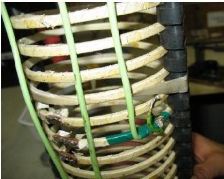
Figure 5. General view of low voltage winding with soldered tap, which brings additional capacity at whole winding
