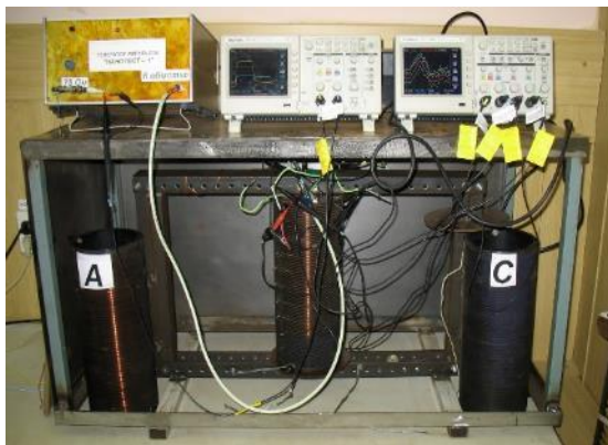
Figure 1. General view of physical model of three-phase power transformer with generator of nanosecond probe pulse and oscilloscopes
