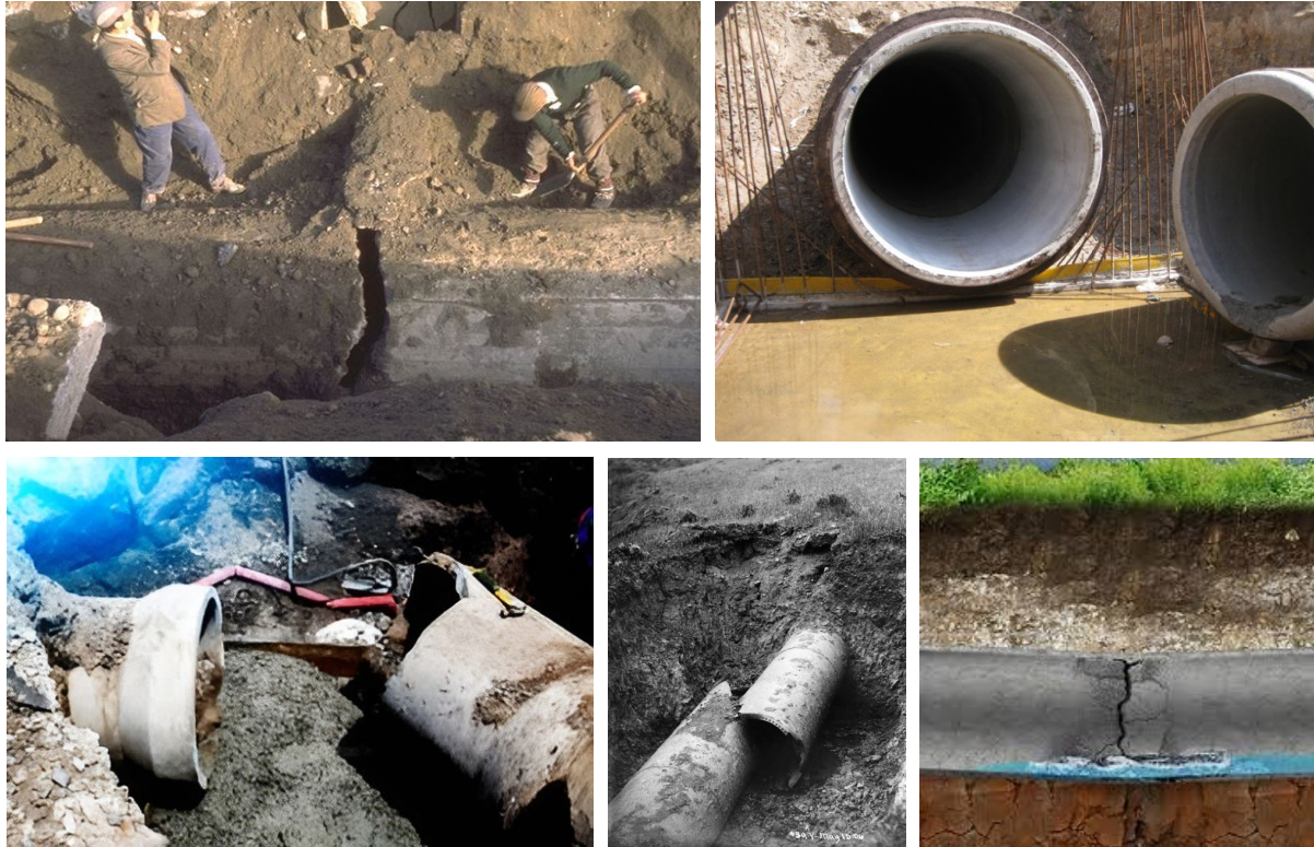
Figure 1. Underground sewer pipe accidents
